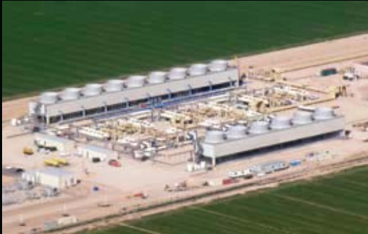
9-Cell & 6-Cell Counterflow Towers - Geothermal
