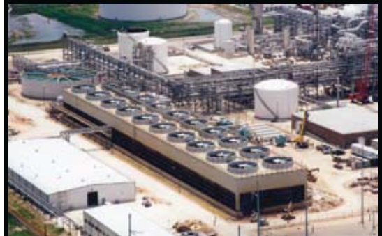
20-Cell Counterflow Tower - Back-to-Back - Refinery
