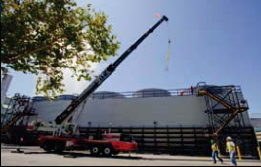
9-Cell Counterflow Tower - Power/Wind Tunnel
