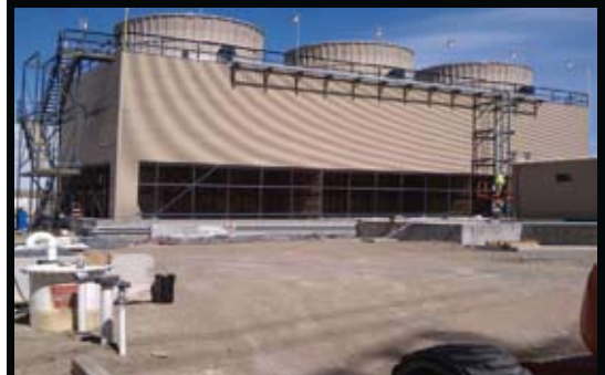
Three 3-Cell Counterflow Towers - Gas-Fired Power
