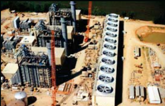
12-Cell Counterflow Tower - Gas-Fired Power
