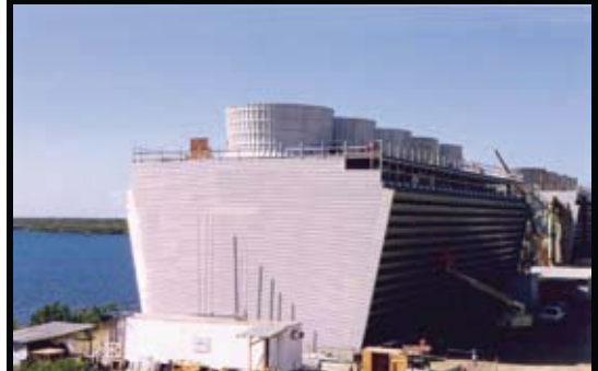
Two 5-Cell Crossflow Towers - Seawater
