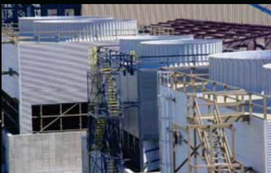
Nine 2-Cell & One 4-Cell Counterflow Towers - Steel Mill Tile Fill/Low-Fouling/Splash Fill - FRP and Wood
