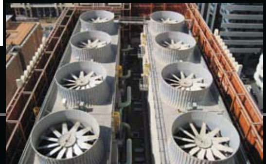
Two 4-Cell Counterflow Towers - Rooftop HVAC Automated-Plume Abated - United Arab Emirates
