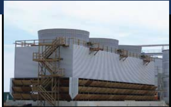
3-Cell Counterflow Tower - Ethanol
